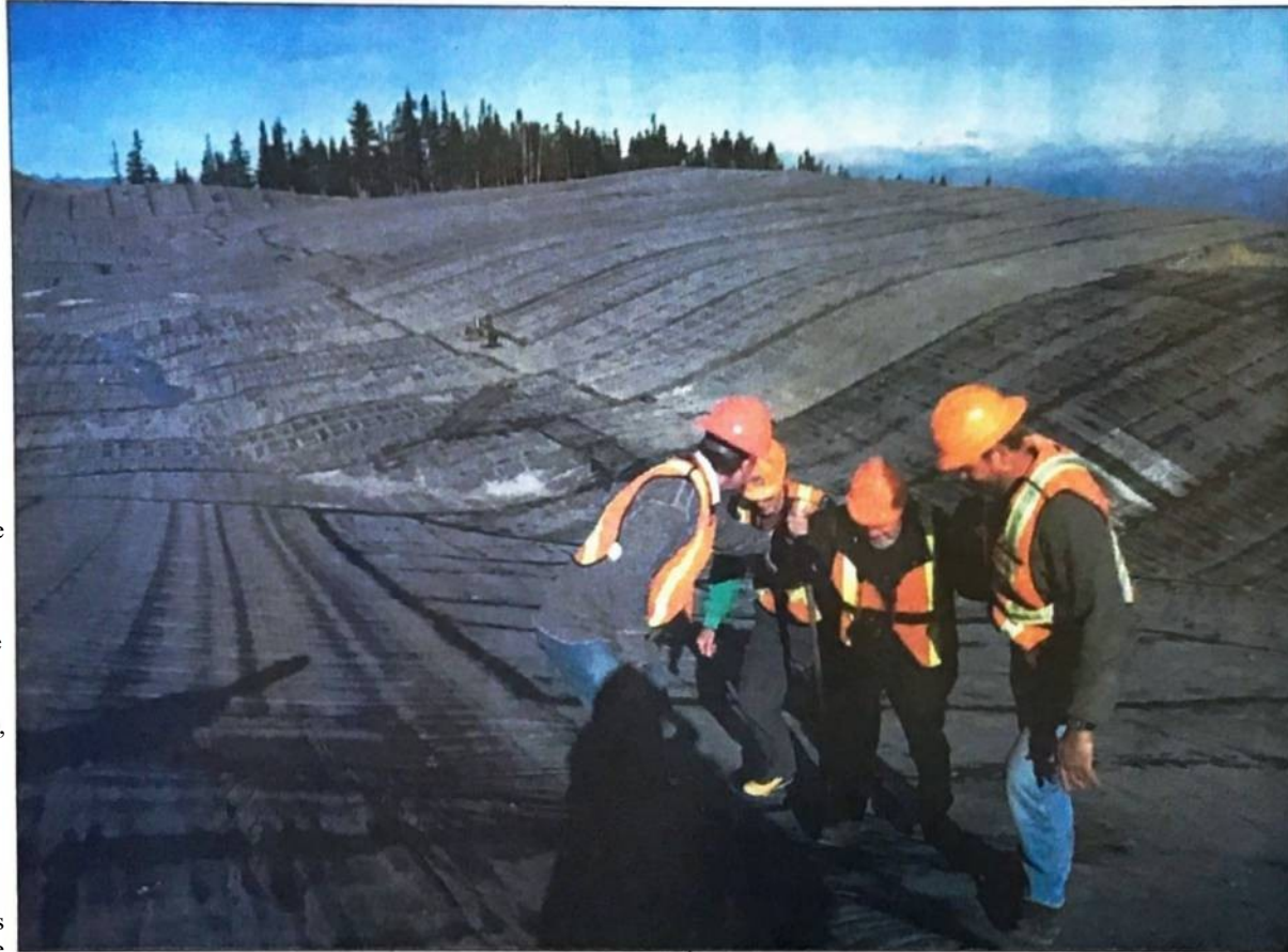
Tsolum River Restoration Society and partners visiting the mine site in 2009 when the cover was complete
