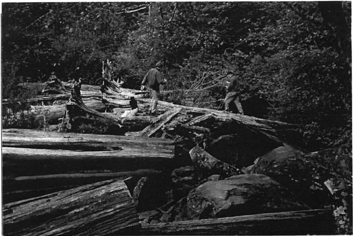
Figure B.2. Weir at Wolf Lake outlet, prior to weir repairs (summer 1998).
