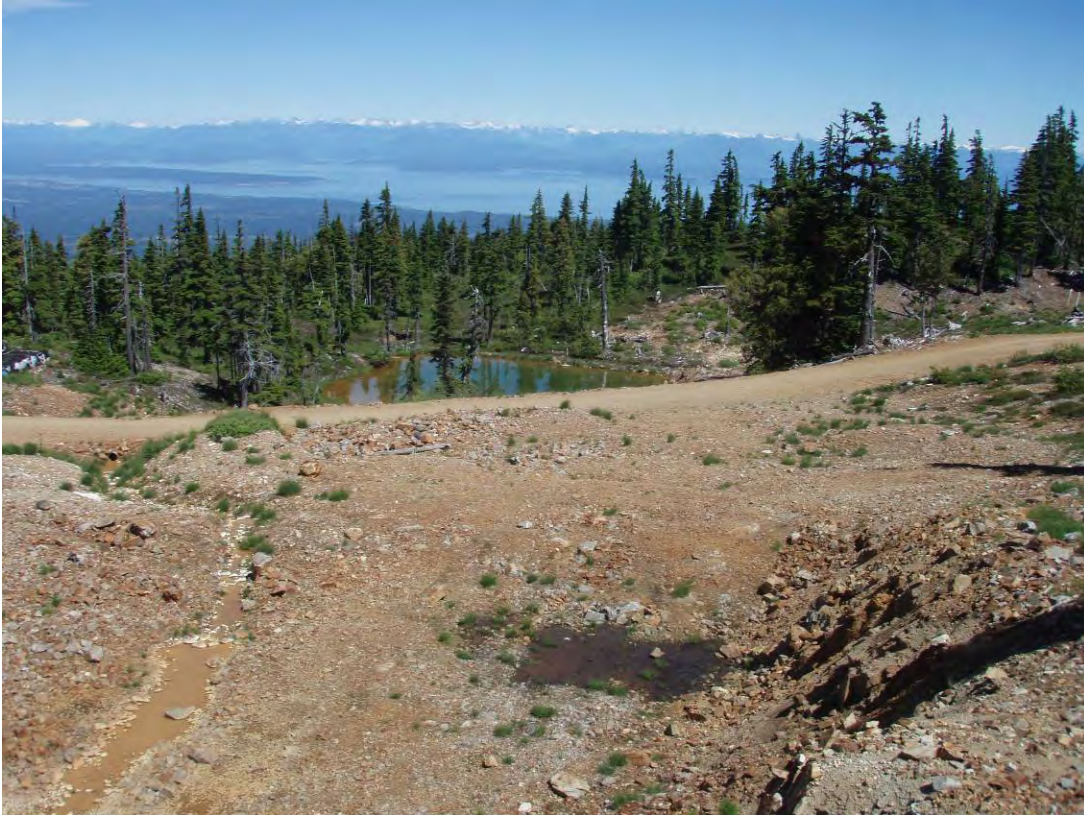
Photo 17: Seepage from Seep 2 to culvert into Dry Pond.
