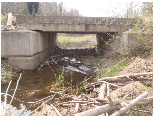
Photo 20. Downstream bridge crossing marking reach break between Reach 5 & Reach 6 (left). Note beaver dam building activity between bridge abutments. (April 4, 2014)
