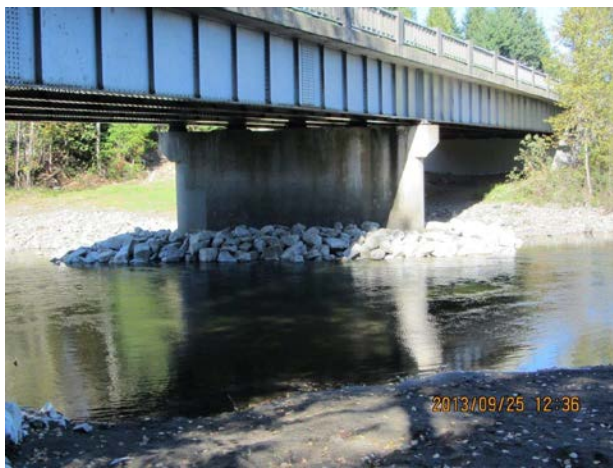
Photo 2. View south (towards the right bank) of the Highway 19A bridge crossing showing rip-rap armouring at the base of bridge abutments that have caused channel narrowing approximately 60 m downstream of the Connolly Sidechannel. (Sept. 25, 2013) (Source: Doug Swift)
